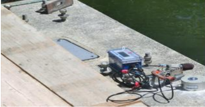
Seismograph geophone secured to the concrete foundation on the 100-year old concrete dam
