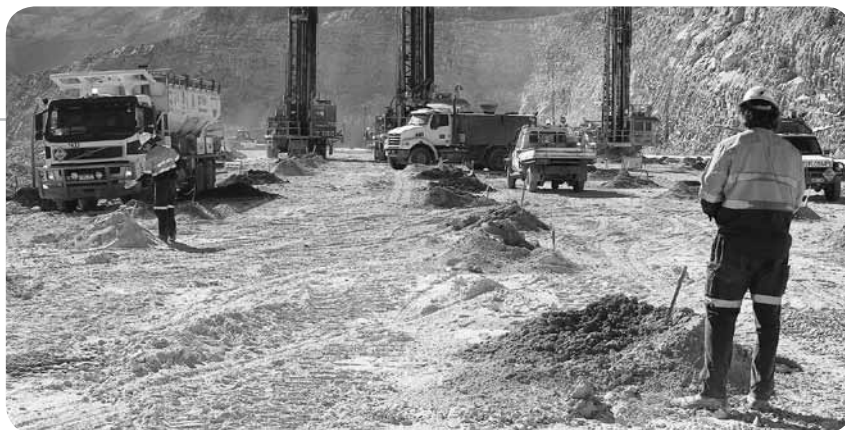
The DNAP team priming holes with boosters, detonators and leads on a mine site.
